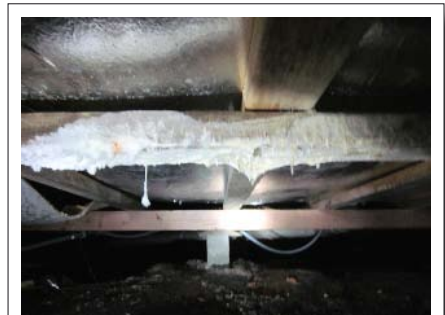
STYRENE/FOIL BETWEEN JOISTS & FUNGAL GROWTH ON BEARER
