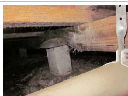
BEARER ROTTED & SLIPPING
