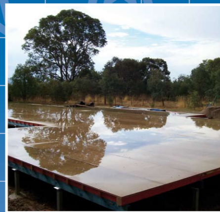
DRAINAGE FROM RAIN
