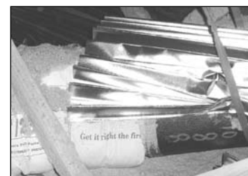
protects cooling ductwork
