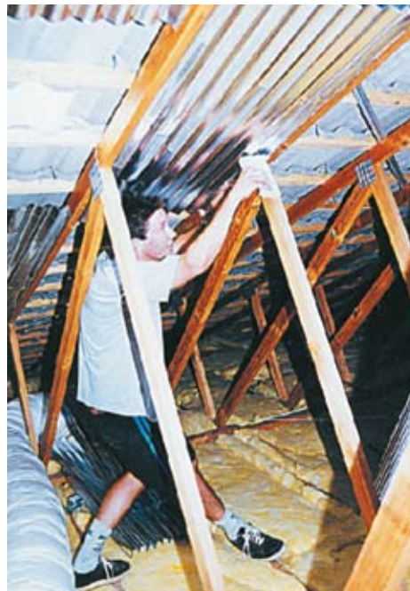
Concertina FOIL BATTs stapled between rafters protects air-conditioning ductwork from intense heat radiating from the roof
